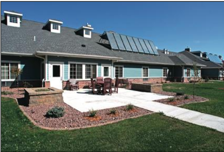
The Pine Ridge Colby facility (above) uses a solar thermal system to provide hot water to its in-floor radiant heating system, working in conjunction with the two Munchkin condensing boilers. The 16 solar collectors can be seen on the facility's rooftop in this photo.
