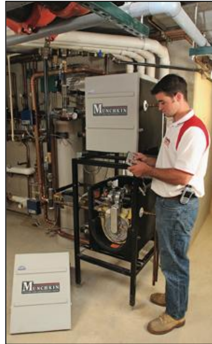
The integrated boiler-management system that controls the two, stacked Munchkin boilers switches from unit to unit to assure equal run times, so that neither becomes the workhorse of the system.
